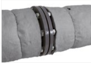
Figure 30: Insulate close to flange, note clearance for bolt removal may be required.
