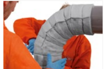
Figure 37: Push all gores together to ensure there are no gaps at joints and tighten wires.
