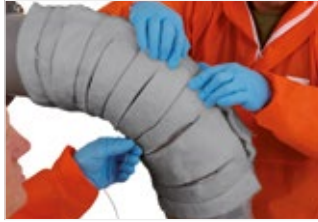
Figure 40: Push all gores together to ensure there are no gaps at joints or voids.
