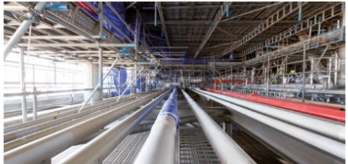
Figure 9: If adverse weather is likely, provide cover for work areas. Prevent insulation becoming wet.
