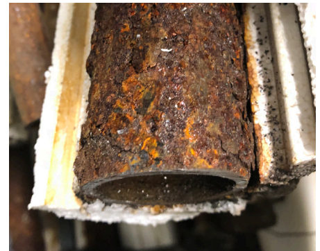
2 A pipe that has corroded due to excessive moisture exposure
